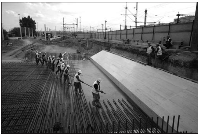
Fig. 7: Installation of the reinforcement of a cast in situ reinforced concrete slab-bridge, formwork for visible surface concrete
